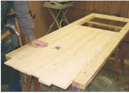
▲ Pic.10 The bead and butt boarding is secured with 38mm oval nails
